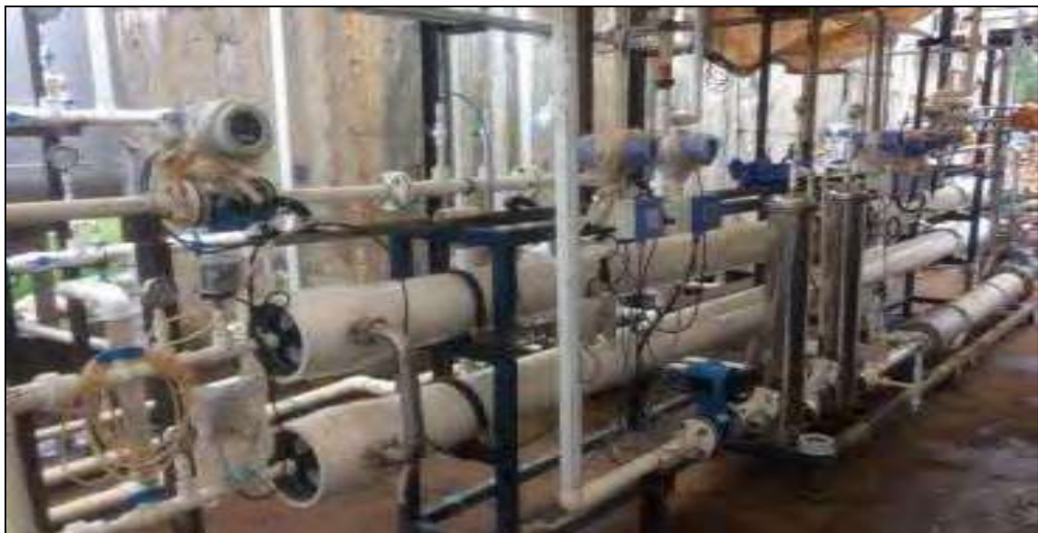
RO based Process condensate Treatment Plan at Distillery
