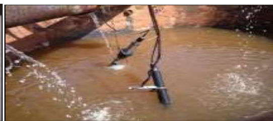
Probe for online monitoring of Treated water quality
